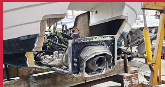
The engine being prepped to install in a Sea Otter 18 at Roudebush Yacht and Engine Works in Dundalk, MD. Photo by Rick Franke
